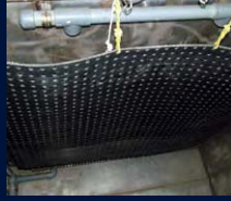
Rubber mats on the wall of the Chilled tank protect fish. The holes are to ensure that circulation is even.
