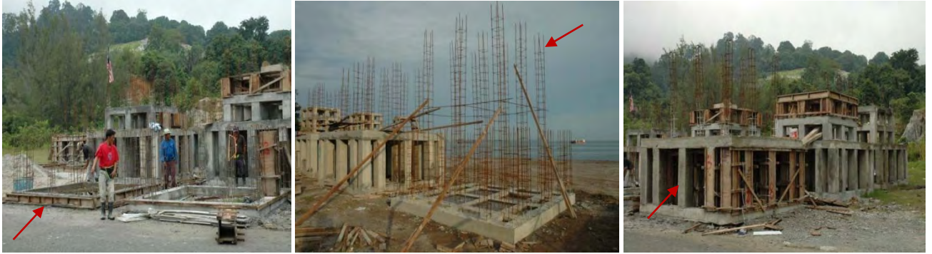
For soft-bottom ARs: construction of base (left), construction of solid steel bar 1.2 cm dia (center), and construction of 25 piles (right)
