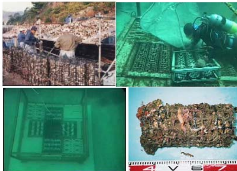
Procedure used for installing test pieces of oyster shells on artificial reef
