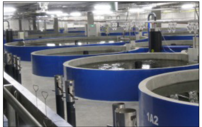
Industrialized Fish Farming Facility
