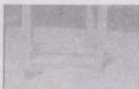
erosion can be observed under corner
