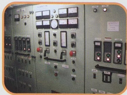
▲ Main switch board
