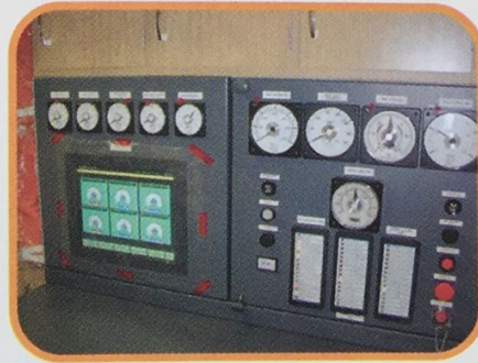
▲ Engine control console
