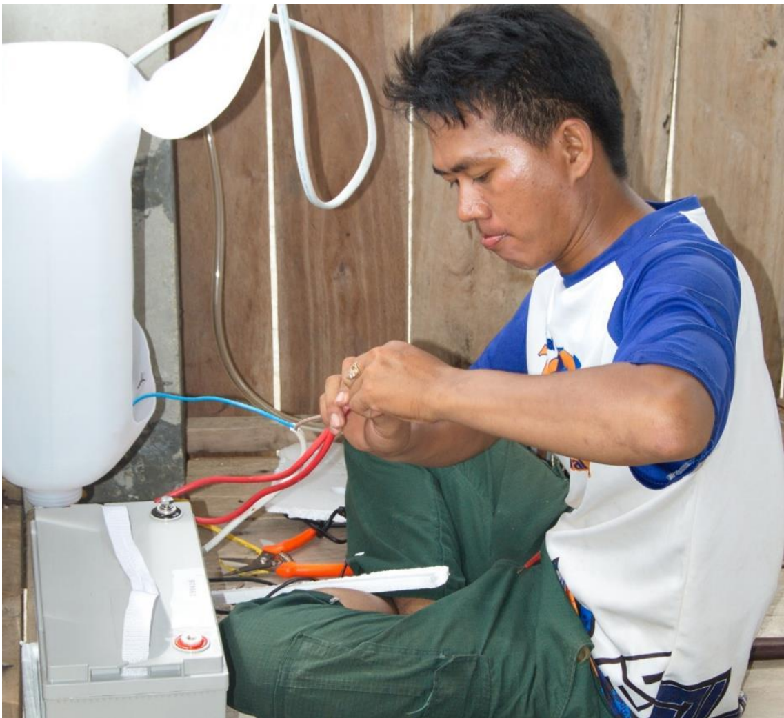
Figure 35. New battery system for solar cell system setting (June 2019)
