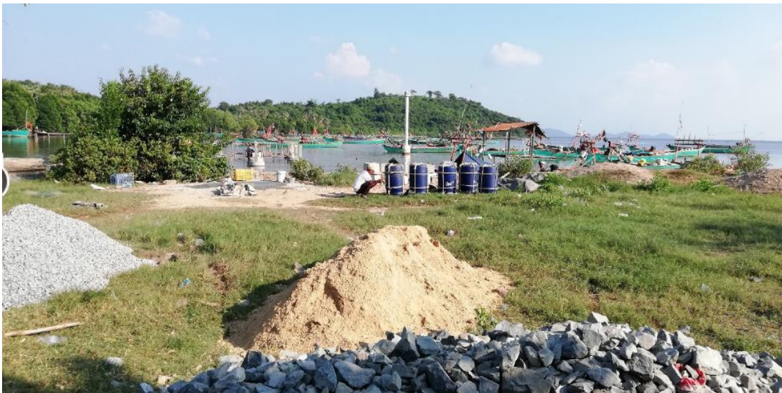
Figure 75. Complete of 12 sets of conservation buoys
