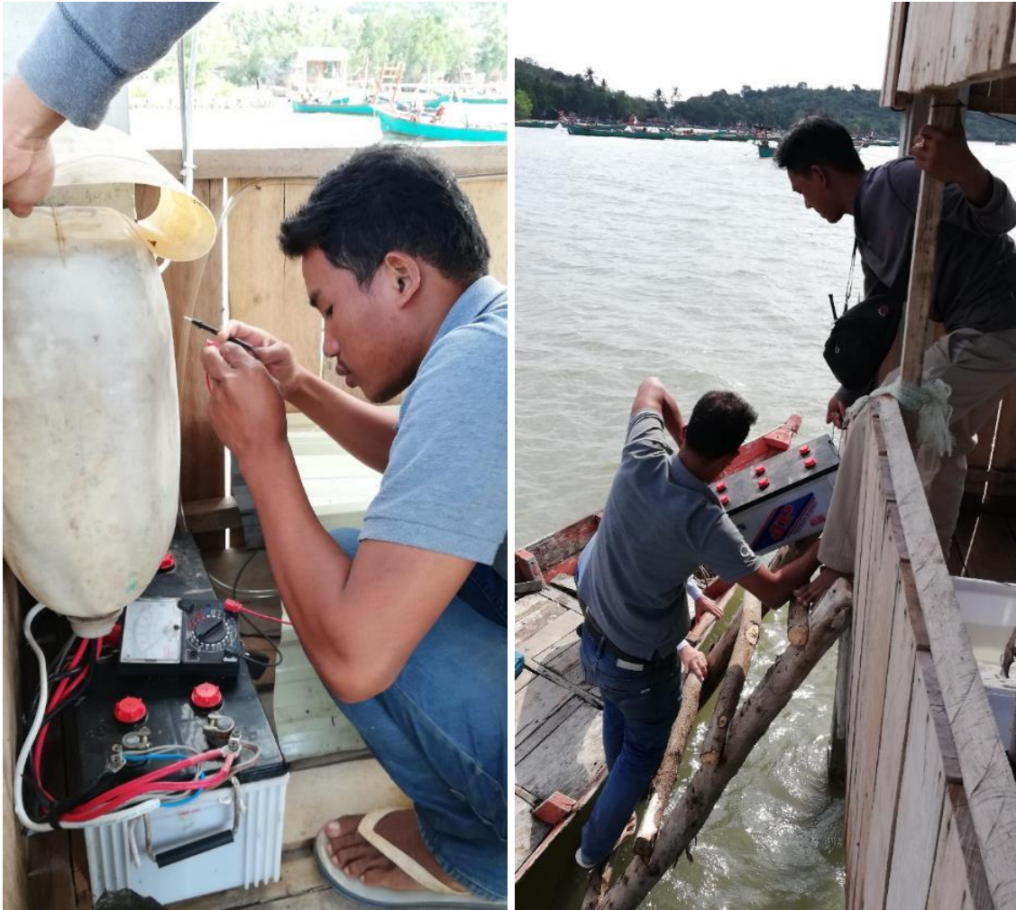
Figure 16. Checking for solar cell and battery system (Left) and battery transfer (Right) (February 2019)
